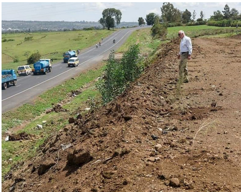
Transformation of the Giotto Waste Disposal Site. Photo credit: Elmad Ogara - County Government Nakuru.
