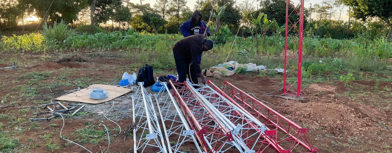
Rural technicians assembling communication towers to bridge the digital divide in Sipili town, Laikipia County
