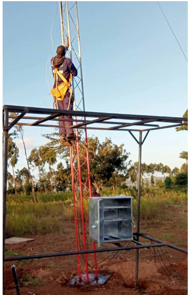
A technician assembling a communications tower mast on top of a hill near Sipili Town, Laikipia County - Kenya.
